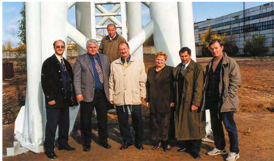
Presentation of UST Track Structure stand under construction to First Deputy Minister of Transport of the Moscow Region Mr. Andrey Kokurin. Ozyory, Moscow Region, October 2001
