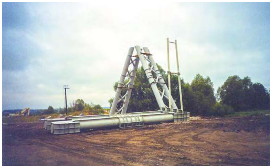
Installation of assemblies for the second anchor support at the UST Track Structure stand under construction. Ozyory, Moscow Region, August 2001
