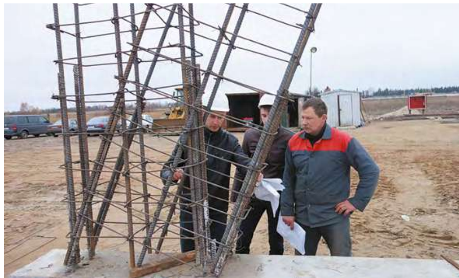
Construction of the pylons of the first high-speed anchor support SkyWay. EcoTechnoPark, Maryina Gorka, November 2015
